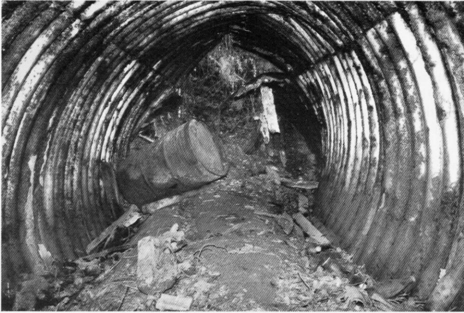
Looking towards the collapsed eastern end of Ashburnham OB
